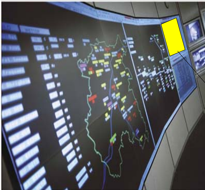
Grid control centre, SWU Ulm
